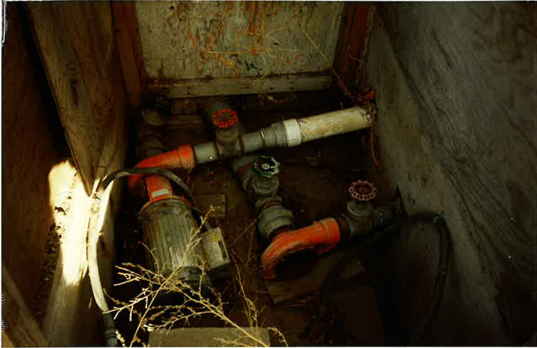
⑨ RELIFT PUMPS - 2 - 20HP BERKLEY'S - NR WELL #2.
