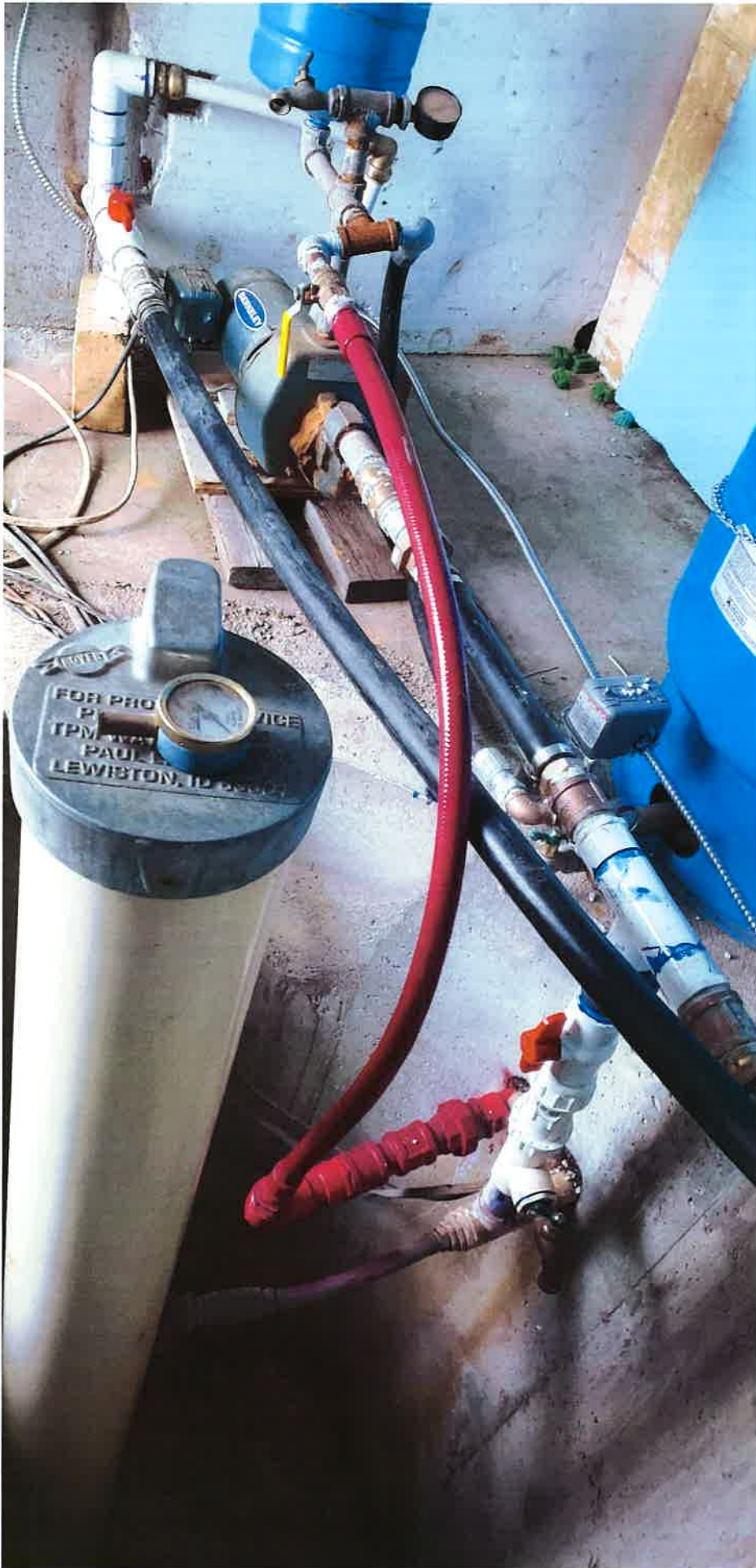
4. Photo showing water line connection to joint water distribution system
