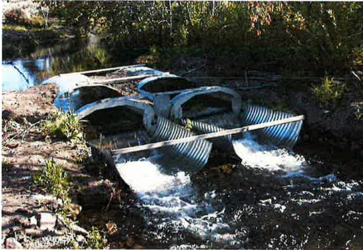
LEFT: View of measuring device, two 42" rectangular weirs, in ABC Agra Upper Diversion Ditch.
