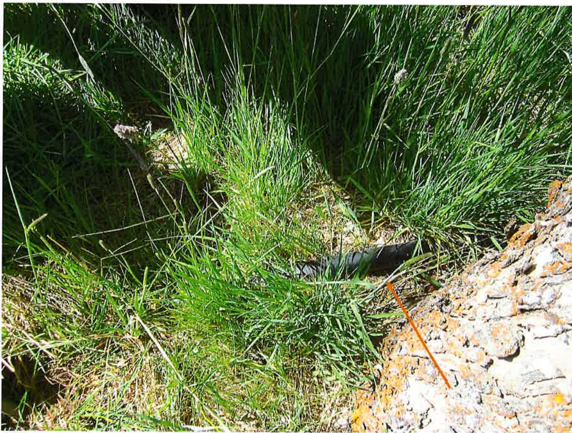
Conveyance method = buried PVC pipeline to spigot for \frac{1}{2} acre domestic irrigation
