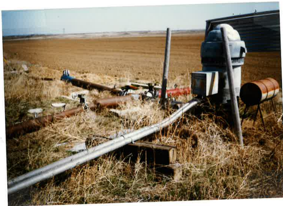
Pump & MAIN LINE SYSTEM
