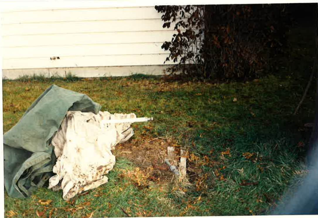
* Sandpoint well located near the southwest corner of the house. (Motor and pump have been pulled for the winter.) This well is used for lawn and garden irrigation.
