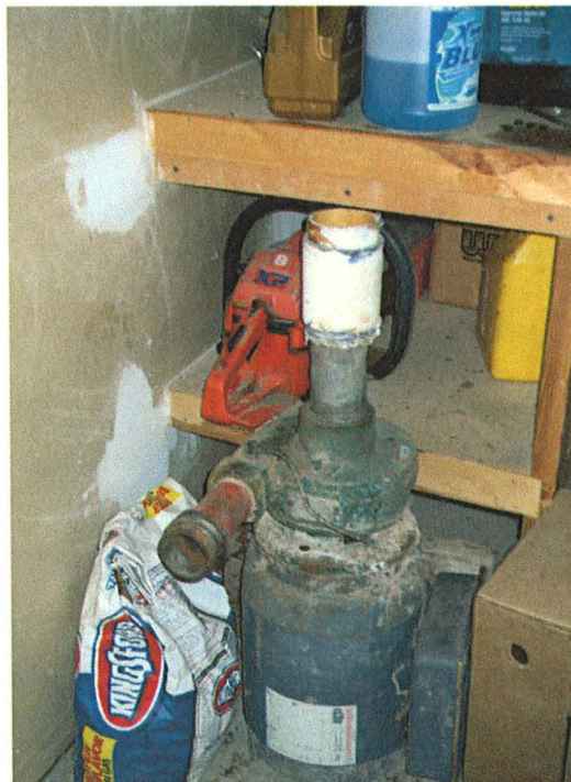
67-4518 10hp pump, currently not in use, is sitting in their shop.
