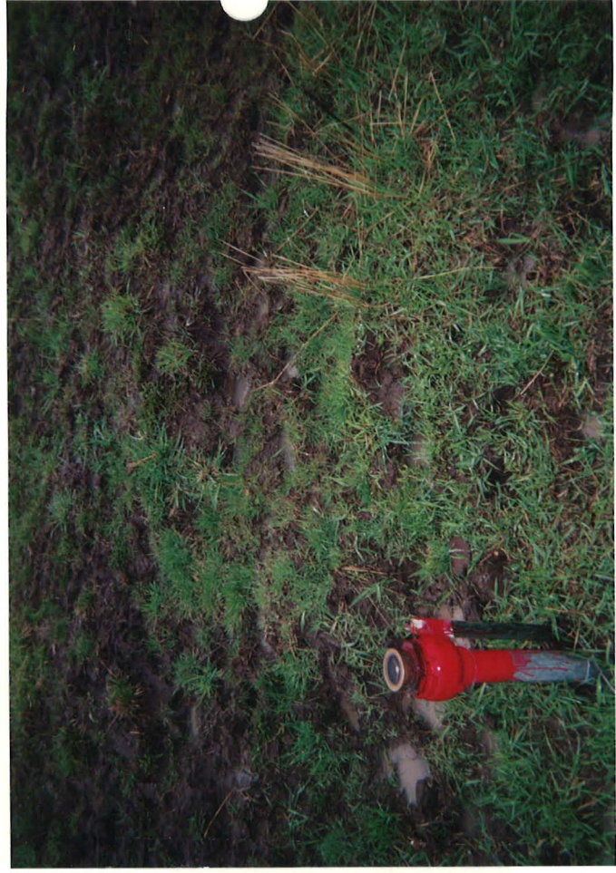
1 of 35 underground sprinkler heads
