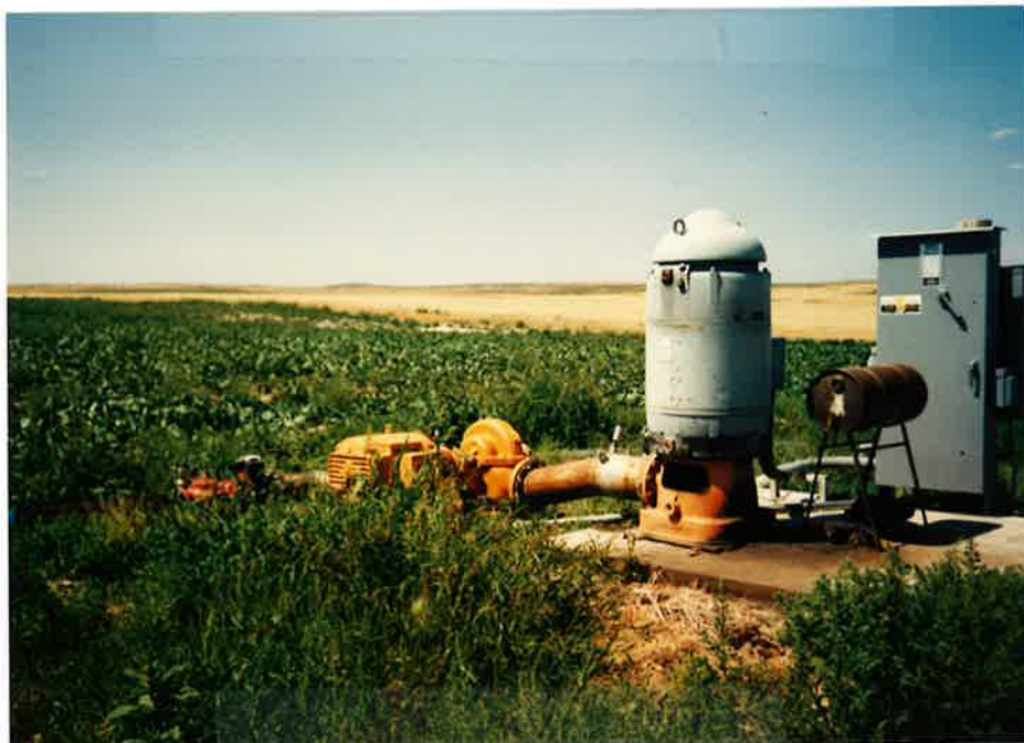
Well & Pump A36-07041 & A36-11340
