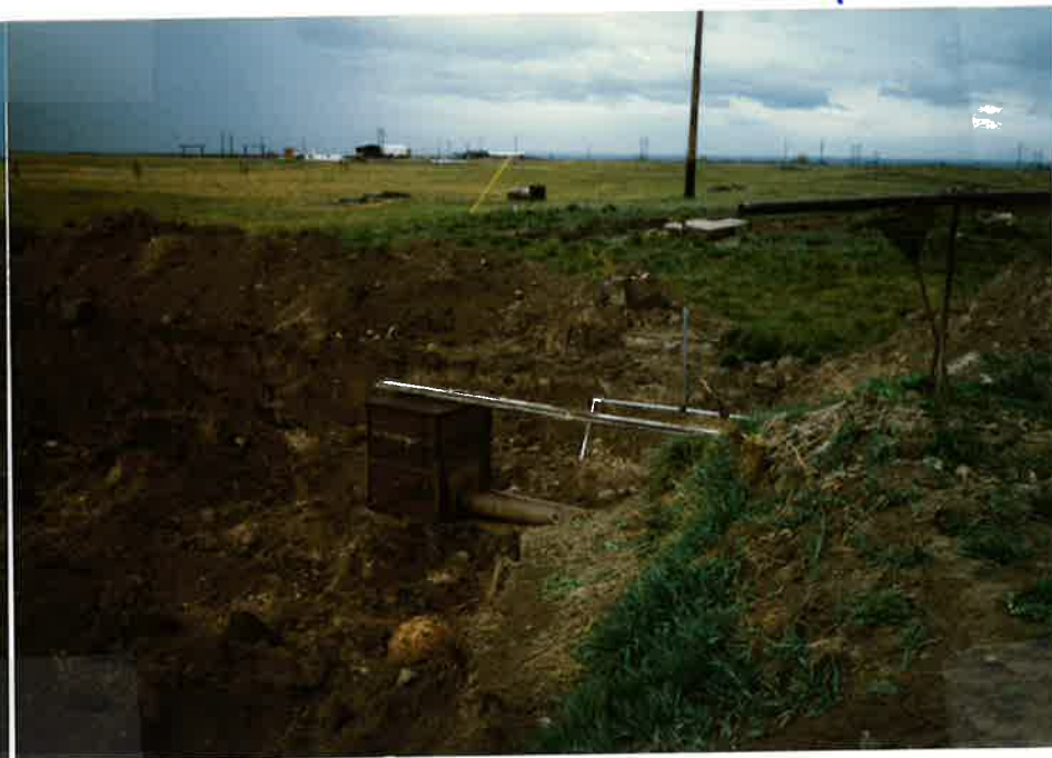
sump + intake To pumps that serve the pivot & mainlines
