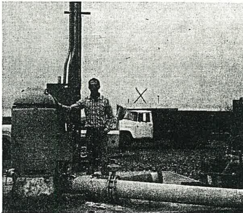
Wayne Maughan shows the rehabilitated pumping plant which has saved about $3,000 this year. To the right the blocked discharge pipe can be seen; a booster pump was located there but was removed after the pump retrofit. (Photo by Randy Lobb)
