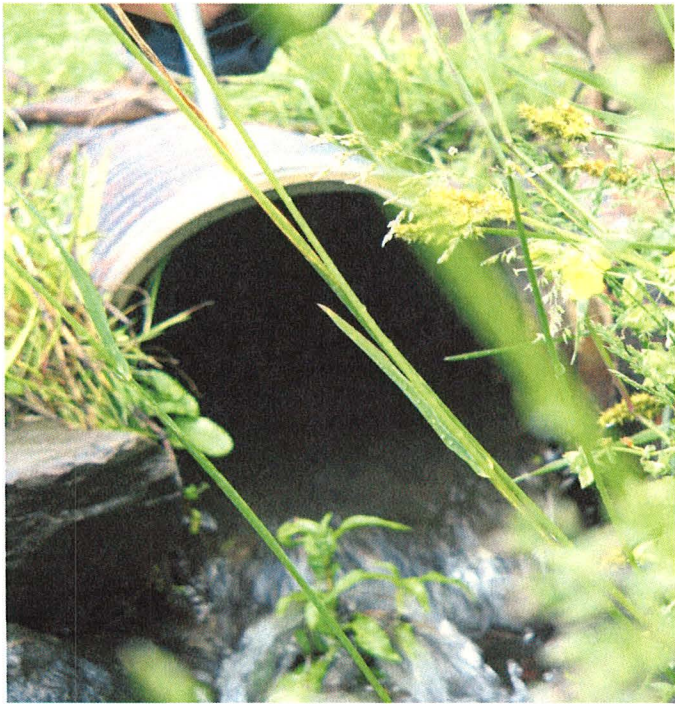
10 inch irrigation pipe carrying spring water.
