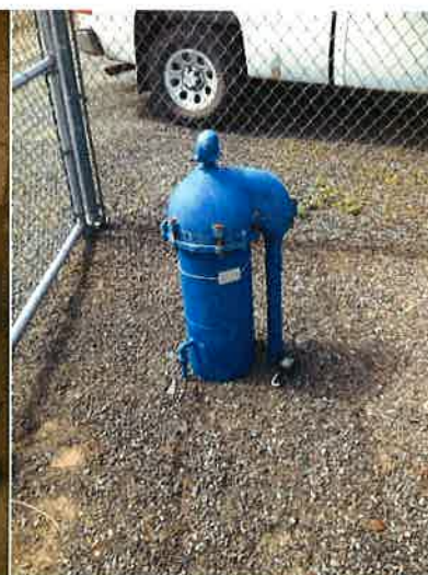
Well No. 5 North Of Town SESW-11-37N-5W
