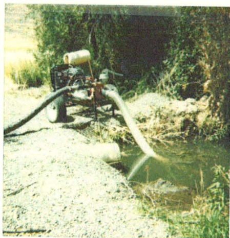
Booster pump from Thousand Springs Cree & portable 7/18/00
