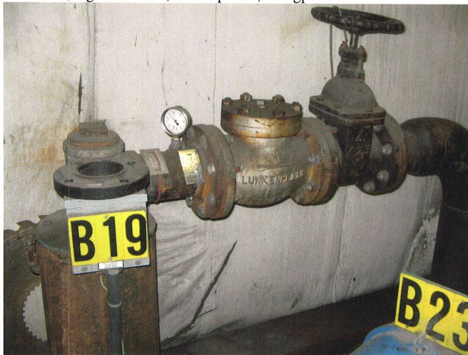
1982 well, originally licensed well, Tag A0017669, 300 gpm.
