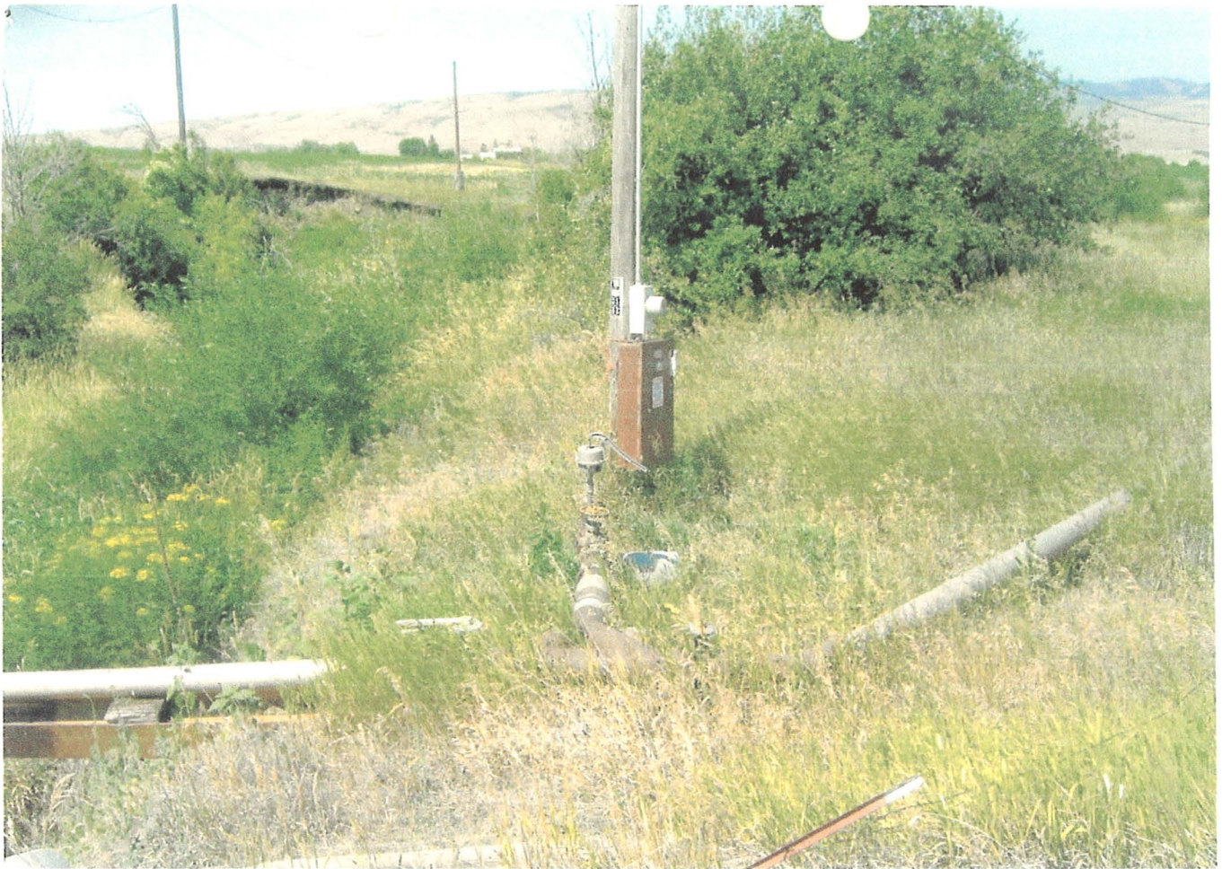
POD 2282476 - 1482342 Pump to MAIN line to wheel lines
