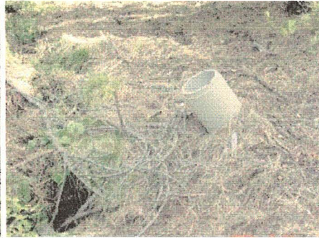
Concrete pipe contains valve controls that regulates water diverted to FS trough pipeline
