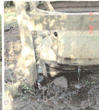
Trough overflow pipe disconnected; drain plug out at bottom of trough, water draining under tank.
