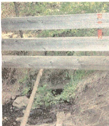
Pipeline from Cistern to FS Trough
