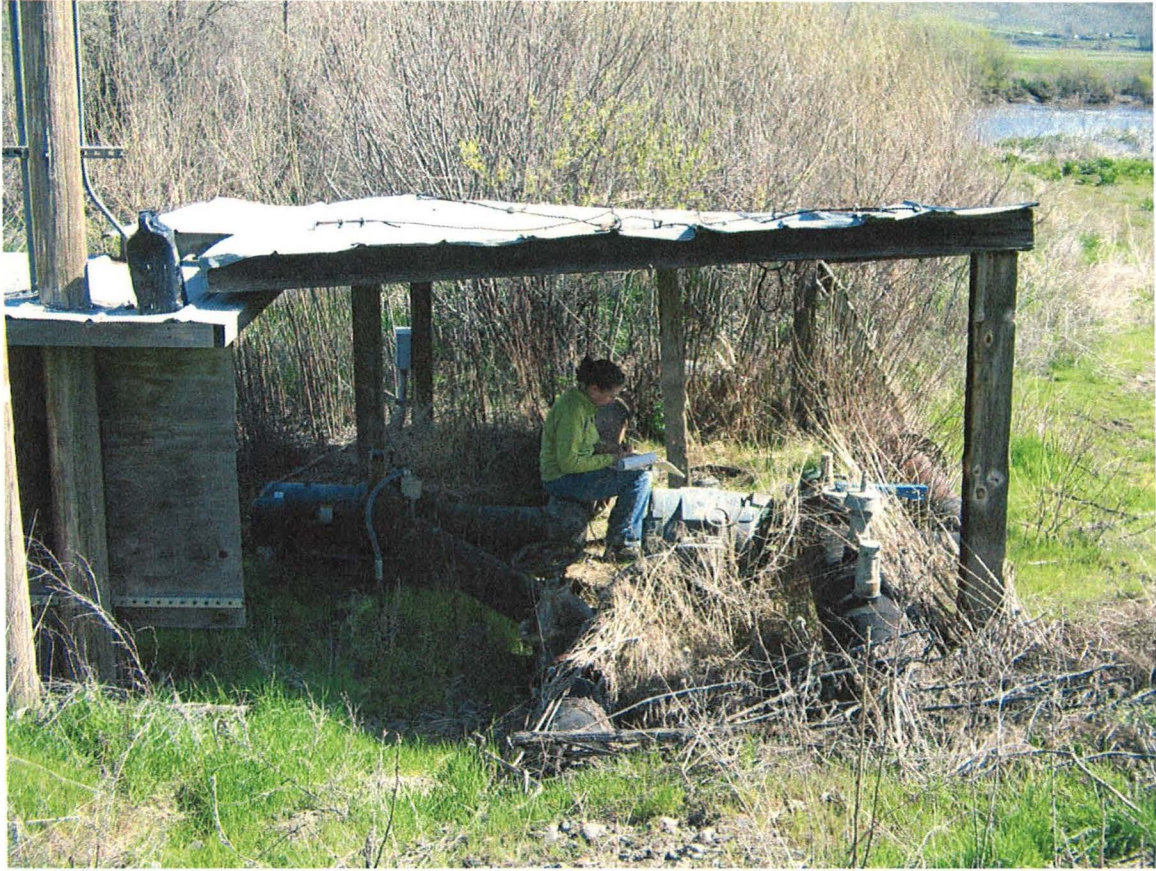
Nevitt Farms POD. GPS Tag A0008994. This is locally known as stations 1 and 2. The two pumps can be seen in the foreground. Weiser River can be seen in the background on the right. The river pumps are put in about where the Weiser River meets the trees in this picture. See complete notes in 67-4504.
