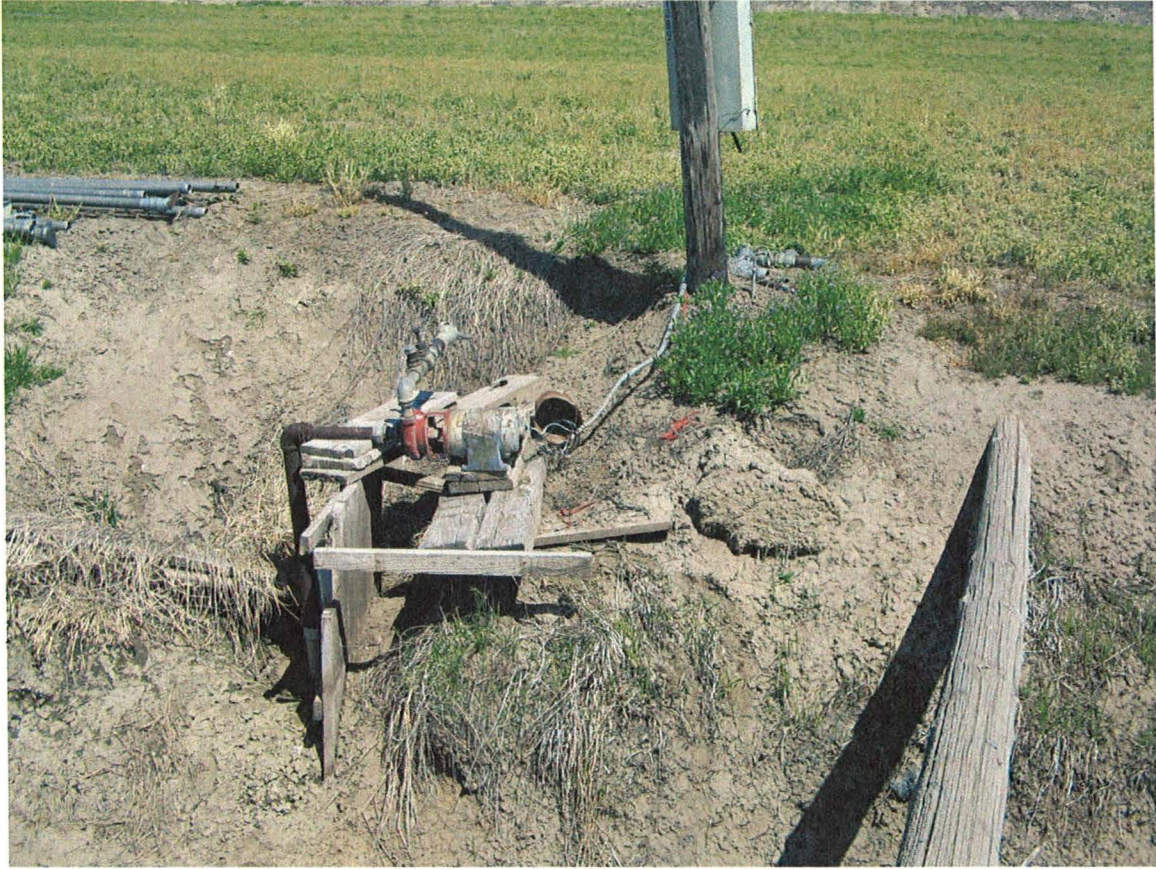
This is the lift station for Nevitt Farms. It irrigates the small patch of ground seen in the background of the picture. This POD is off of Hill Road, just off of Cove Road. This was GPSed but not tagged. GPS coordinates in FE for 67-4504.
