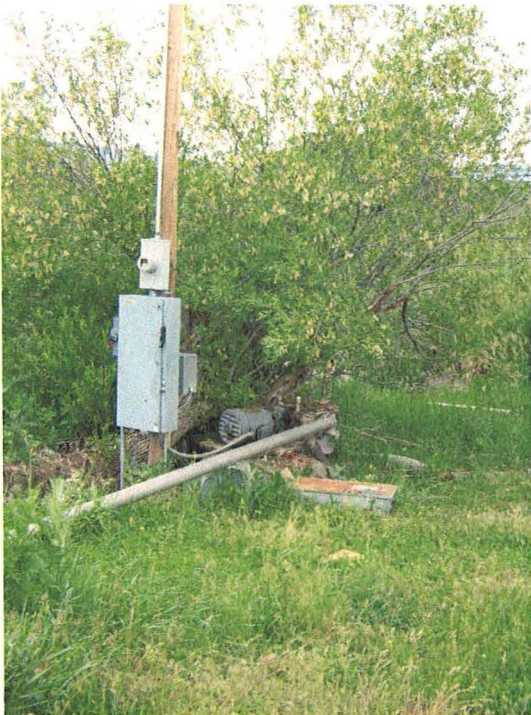
A0017646. Bonner's pump off of Banner Creek. Banner Creek is flowing from right to left in the picture on the far side. The pipe visible in the middle of the picture continues to the southwest, where it goes up and out to the fields as shown in the layout in the file. Photo taken facing north-northwest.
