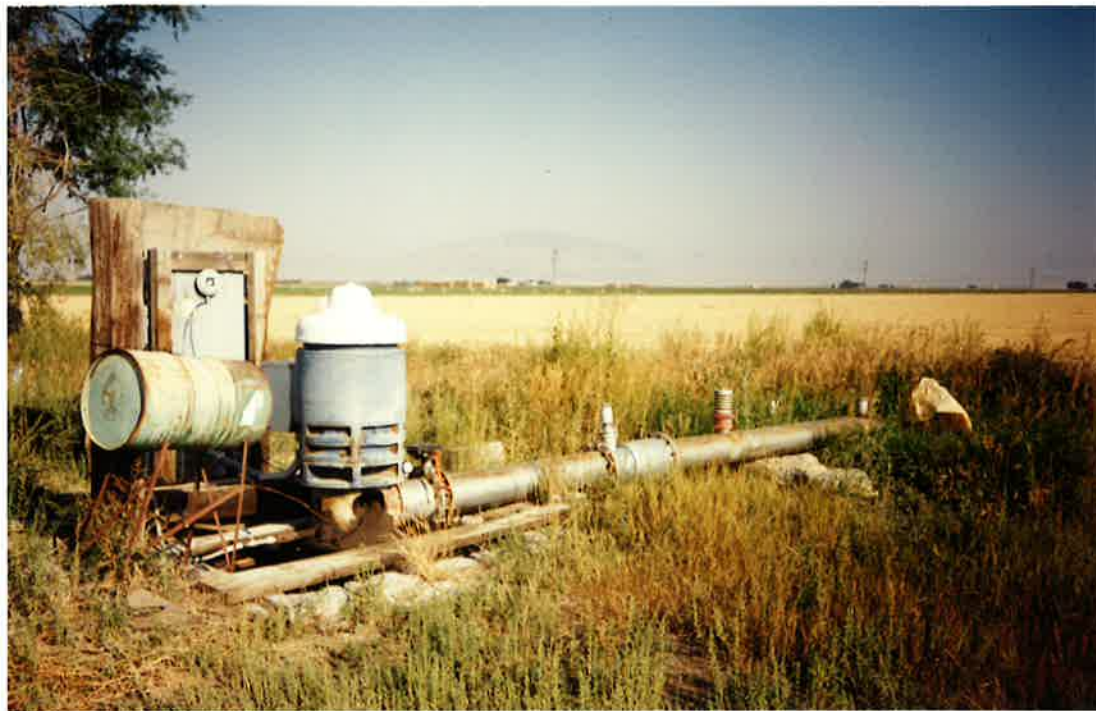
Photo # 1-10 LOOKING NW FROM THE POD IN THE NW SW SW Sec 12 SHOWING THE MOTOR & PUMP
