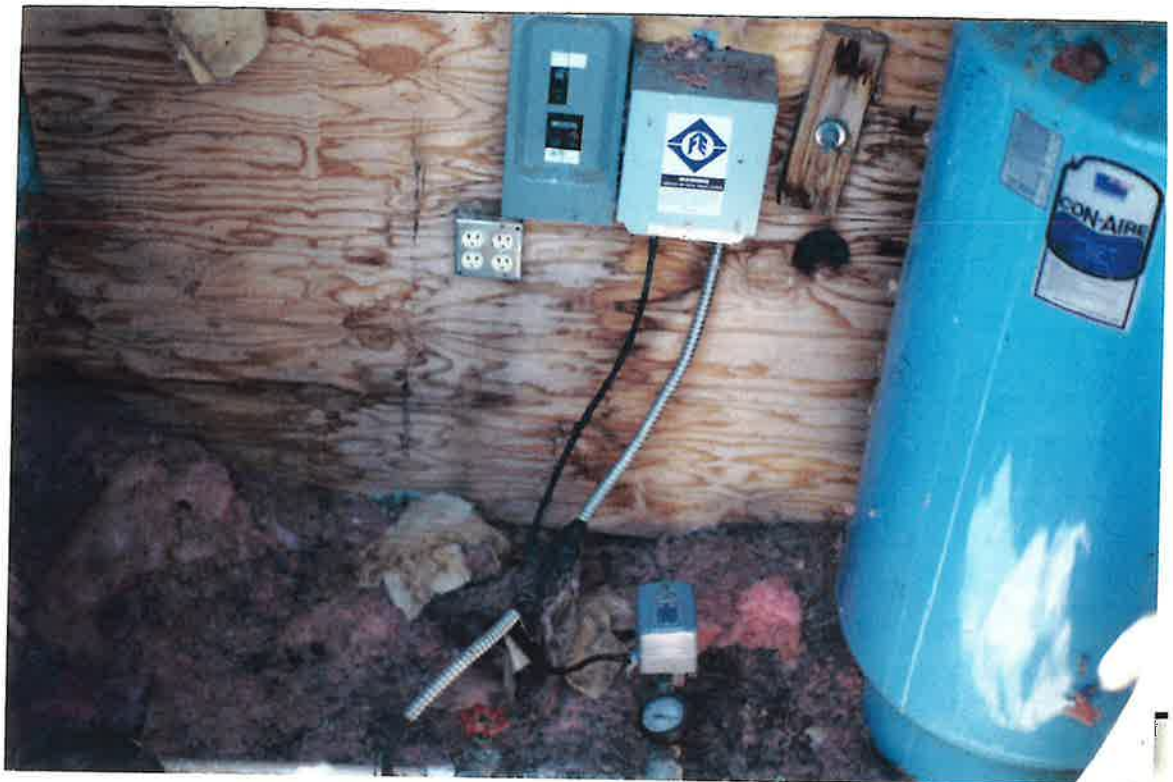
INSIDE WELL HOUSE
