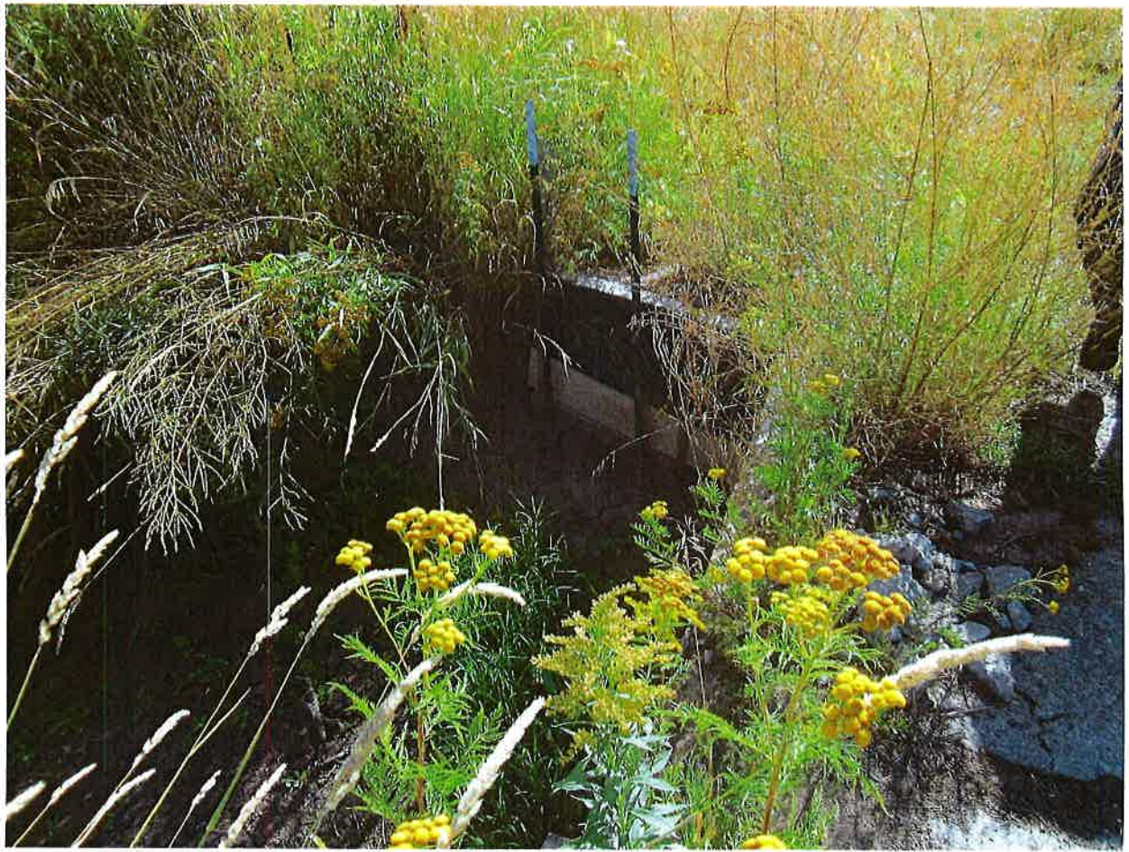
Figure 2- Diversion from creek (next to original culvert) towards south east creating "Flood Creek" which then runs parallel to creek/road southward until about 30 ft. in trees. "Flood Creek" ends about 30 ft. in trees, water flows freely.
