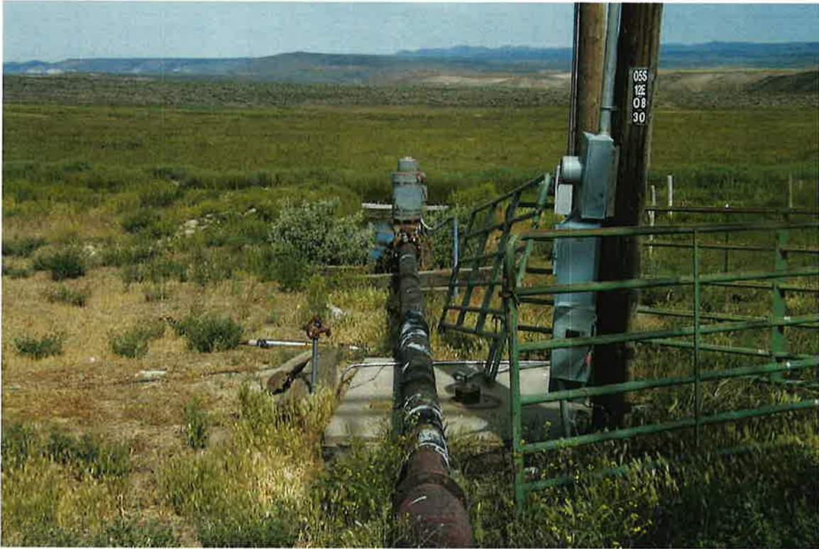
Point of Diversion looking northwest. The irrigation pump has been pulled and only the pump supplying water for 37-10999 is in the well. A 100 HP pump in the ditch is being used to supply water to the place of use at this time. CLF 6-4-02
