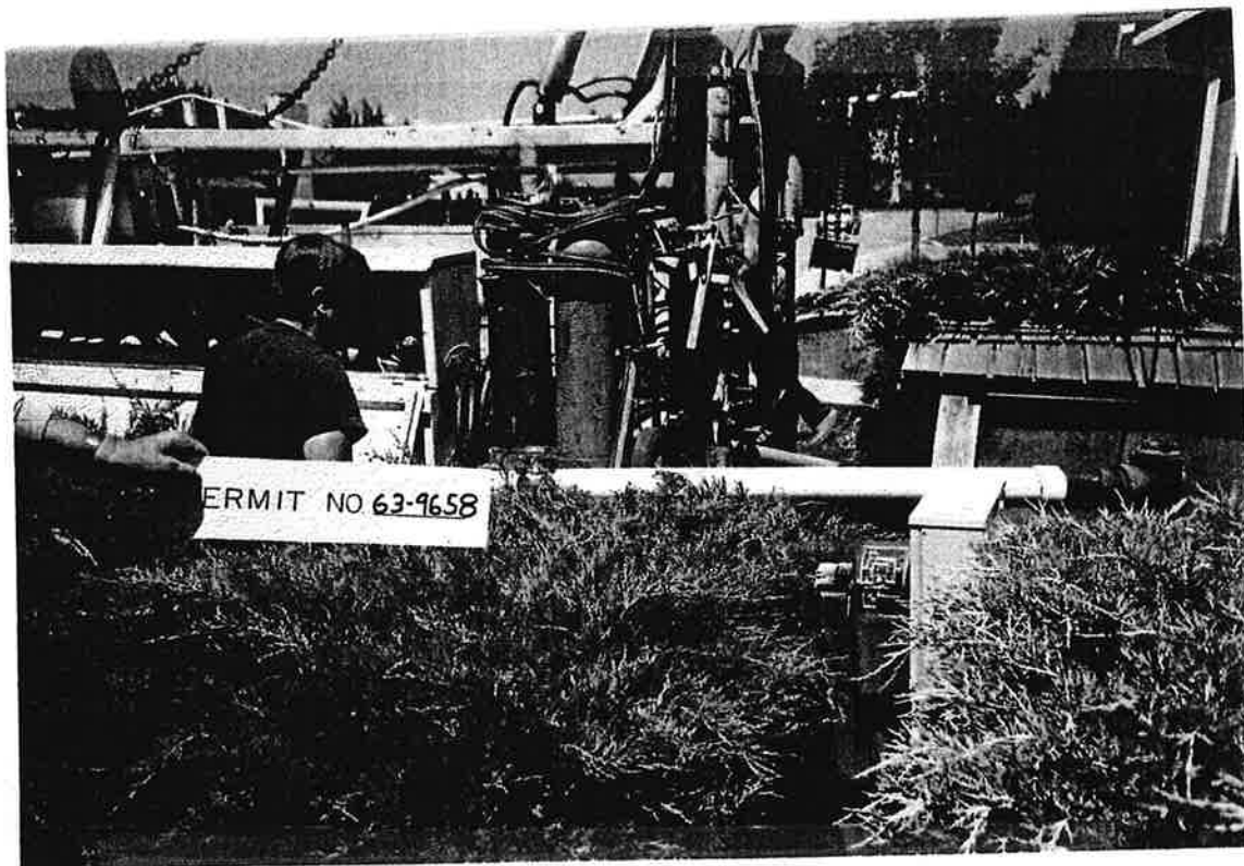
Hayes Pump and generator Men working on vehicle See Permit 63-08402 on Raindrop Drive.
