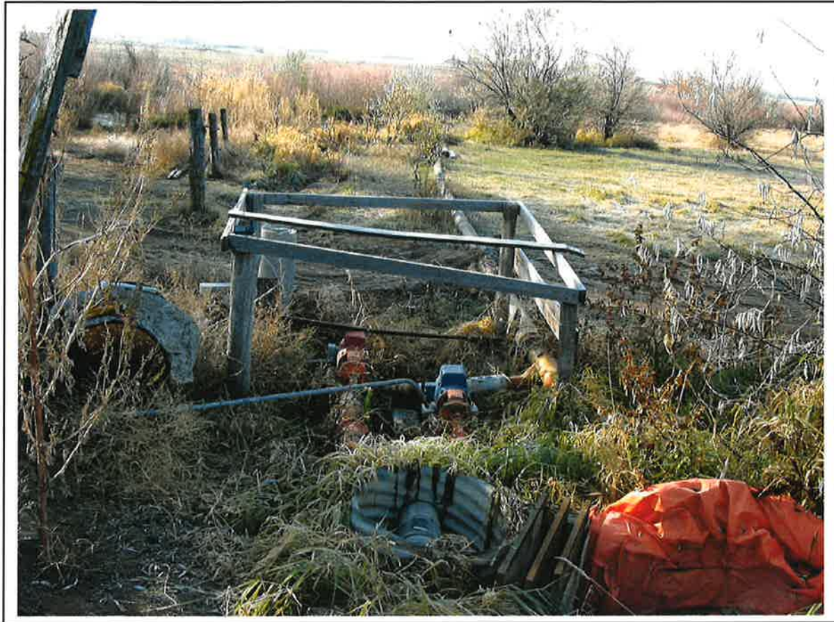
Two 7.5 HP pumps in the Carpenter Ditch on north side of the Big Wood River. Lee Peterson Photo 11-23-04. Photo taken from the north side of the Carpenter Ditch looking south towards the POU that is across the river.
