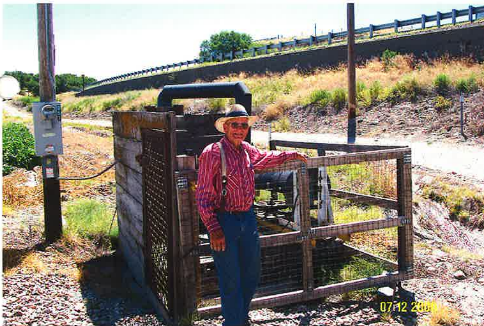
PUMPSTATION PUMP DATA IN FILE
