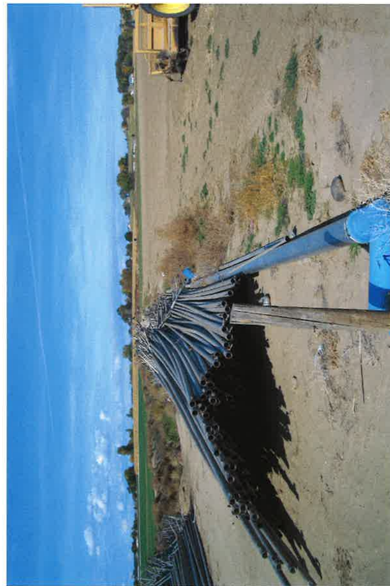
8" main line from pump to NWSF
