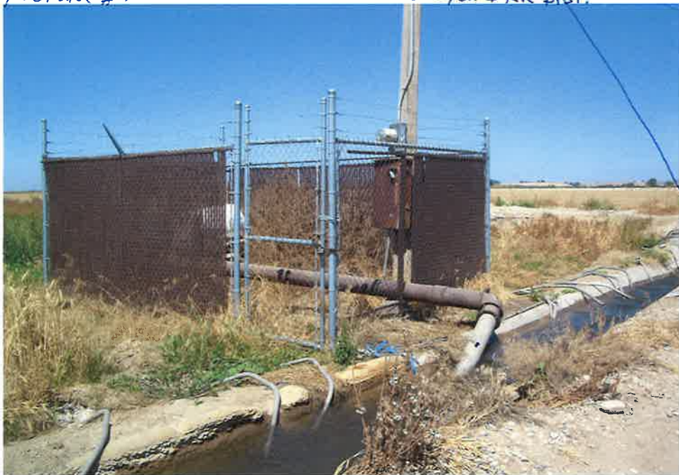
6" Discharge to cement ditch for gravity IRR.
