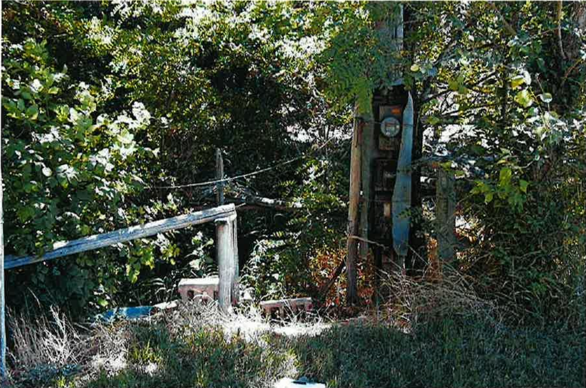
Power box for POD. Looking SE. Irrigated field behind me in picture and Portneuf river straight ahead. (csaxton).
