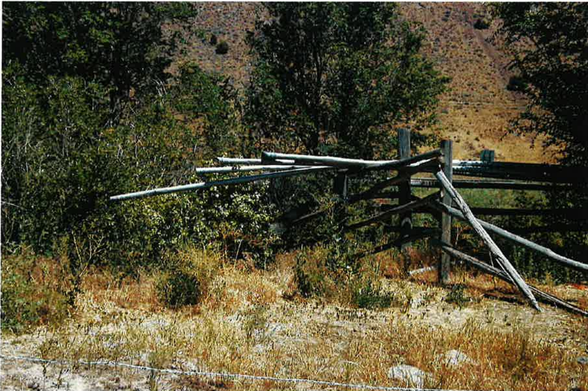
Looking North. This sprinkler pipe is just East of the Pump. Pump is to the left in the picture. Irrigated field behind me in the picture. Portneuf straight ahead (csaxton)
