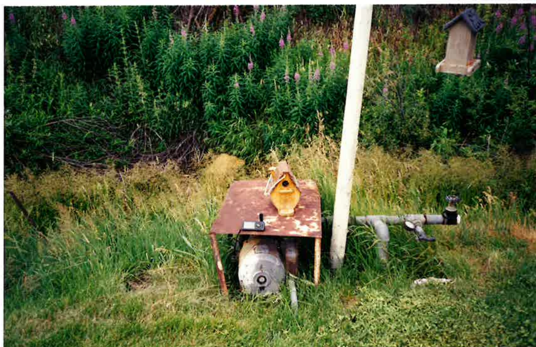
Pump located on Back or West Side of House.
