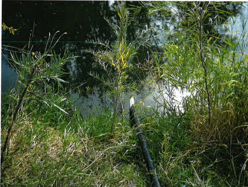
Looking SW at intake line from the Portneuf River. POU behind me in picture.
