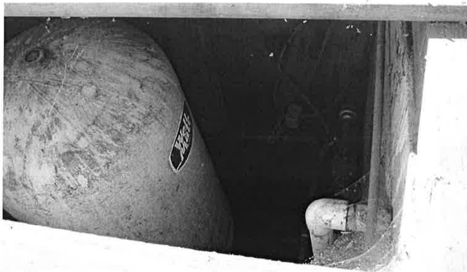
Looking down inside well house.
