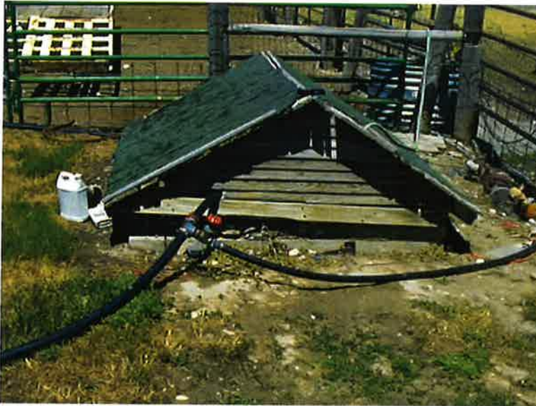
Picture of pump house, facing north.
