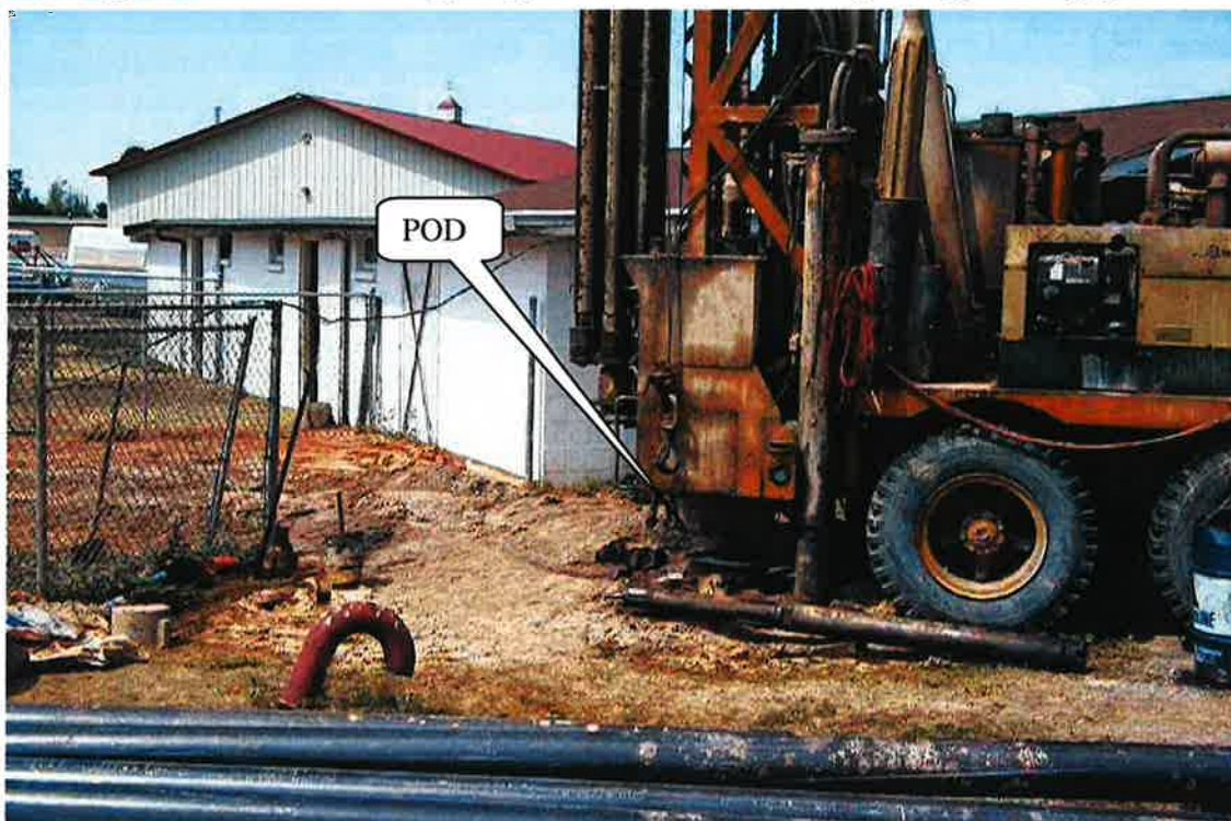
Looking North. Original well located in barn shown in picture. Picture taken while in the process of drilling a replacement well. POU to right and left of picture. (csaxton 8/8/01).
