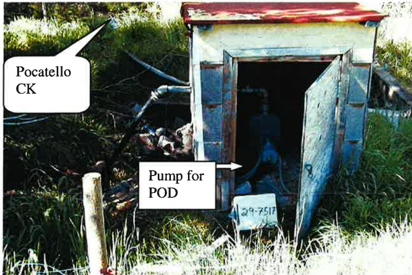
Pump Located on Leo's place but services irrigation for Mr. Hurst's original home. Looking South. Pocatello Creek in background.
