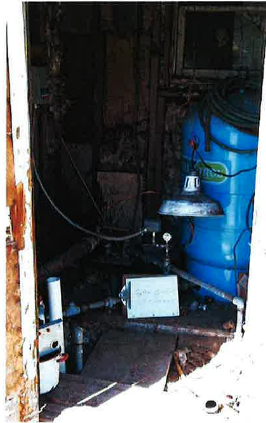
POD Well inside of well house. Two pumps, Irrigation pump is 5 hp and domestic pump is 1 hp. Picture taken 5/4/01 by Craig Saxton
