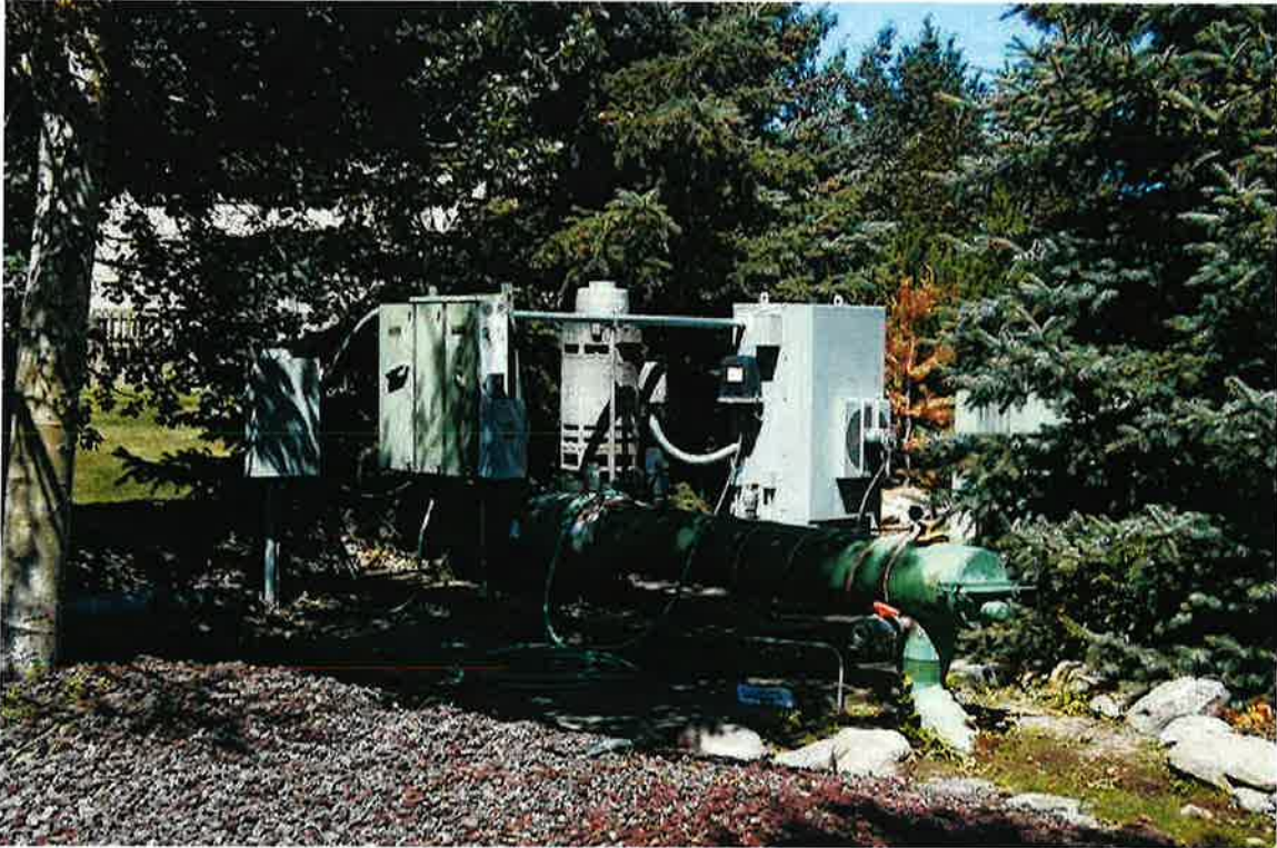
Booster Pump. Looking NW. This is the pump that takes the water from the pond and distributes it throughout the sprinkler system throughout the golf course. (csaxton).
