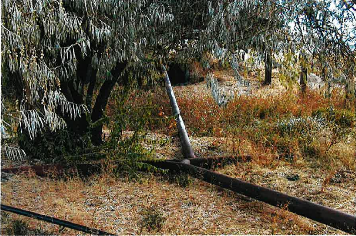
Out take pipes exiting the irrigation well. Irrigation well behind me in picture. Picture taken looking East (csaxton 10/24/01)
