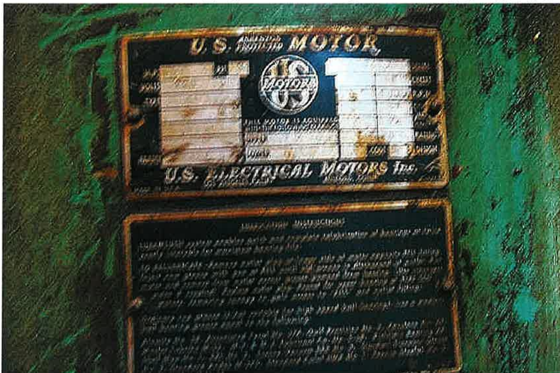
Irrigation pump label. Make us U.S. Electrical Motors: HP - 30: SN - 1059472: Cycles -60 (csaxton 10/24/01).
