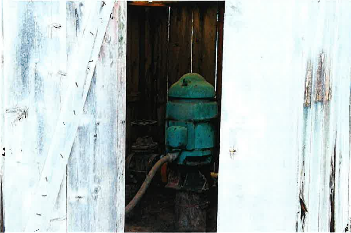
Irrigation well inside well house (csaxton 10/24/01).
