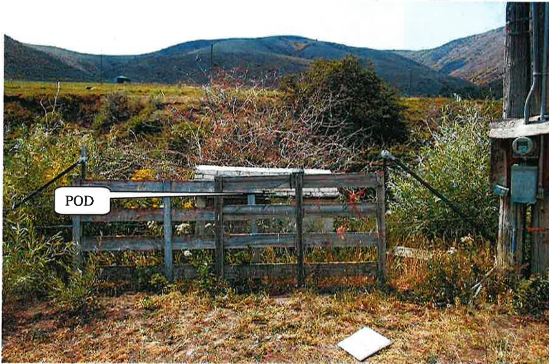
Looking South. Pump is on North side of Portneuf. Irrigated POU behind me in picture. Portneuf below pump house in picture (csaxton 8/21/01).
