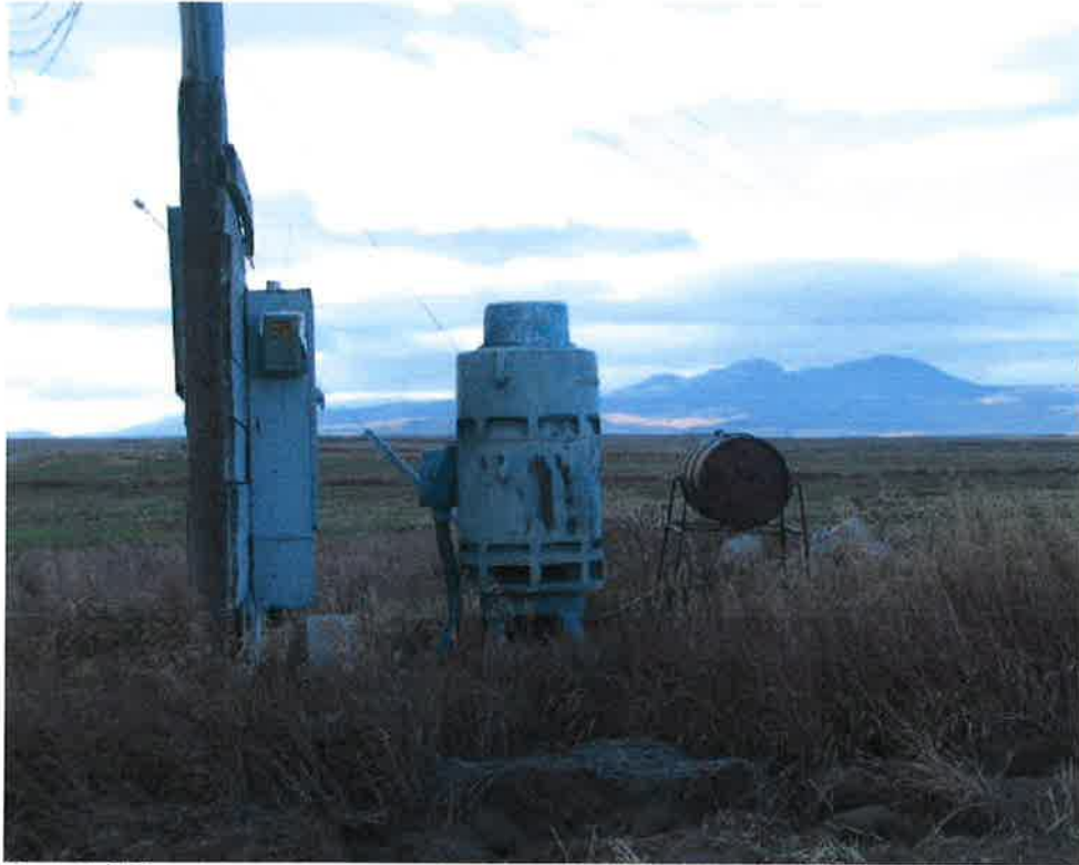
Photo 1. G.E. 125 hp pump, Model 5K505XC024A. Looking northeasterly. (IMG_0182.JPG)
