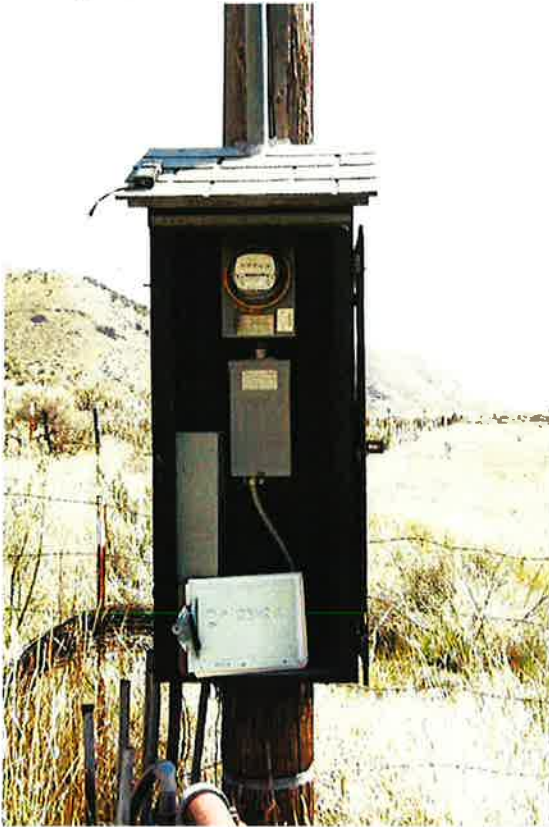
29-02342A Power box installed in 1983. Looking East.
