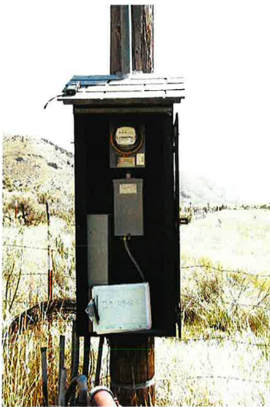
29-02342A Power box installed in 1983. Looking East.
