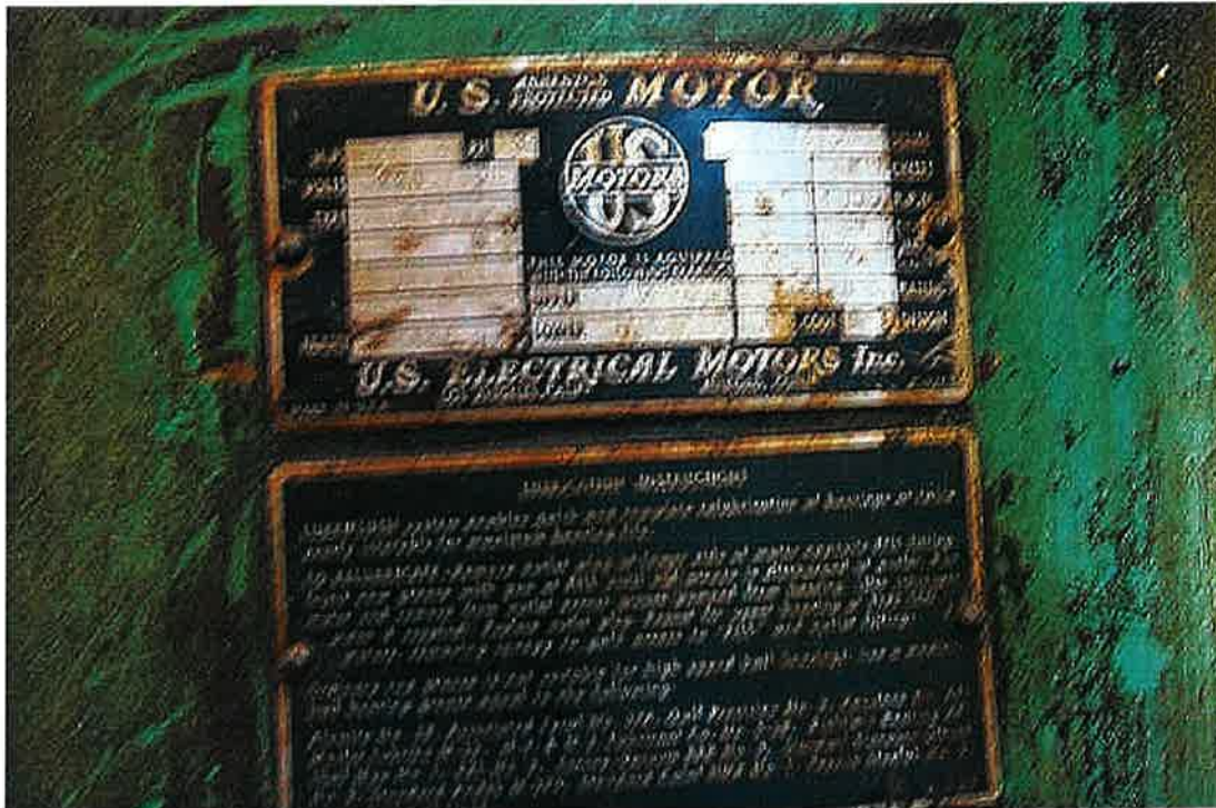
Irrigation pump label. Make us U.S. Electrical Motors: HP - 30: SN - 1059472: Cycles -60 (csaxton 10/11/01).
