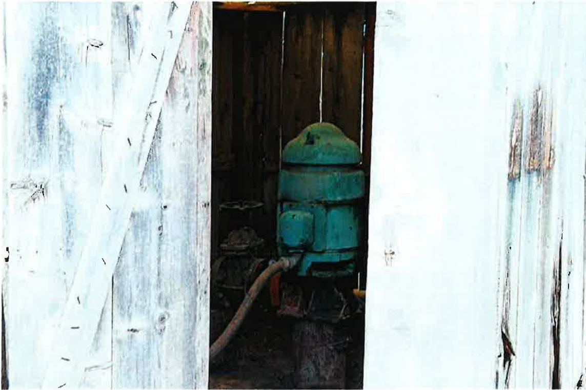
Irrigation well inside well house (csaxton 10/24/01).
