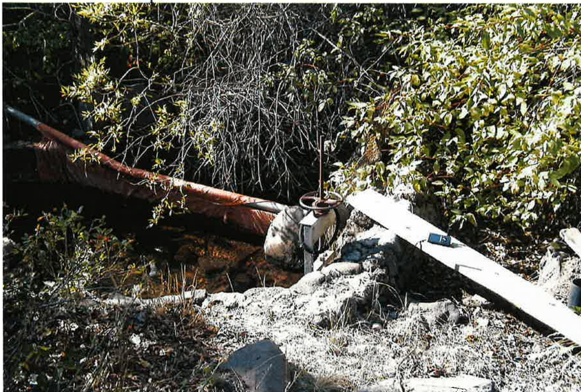
Photo 1. FX Aug. 8, 2001. Photos by RDH. 63-00115: POD located T01N, R07E, S14, SWNENW. Screw head gate, plastic, rock dam diverts into underground 14" steel pipe and risers. POD overlaps 63-31290 & 63-31296.
