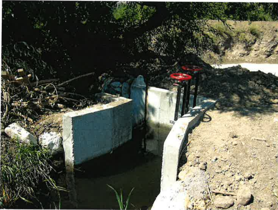
Looking NW at POD for all Indian Creek rights with a POU south of W Portneuf RD. Water is diverted to the right of picture to irrigate claimants Trees (csaxton).
