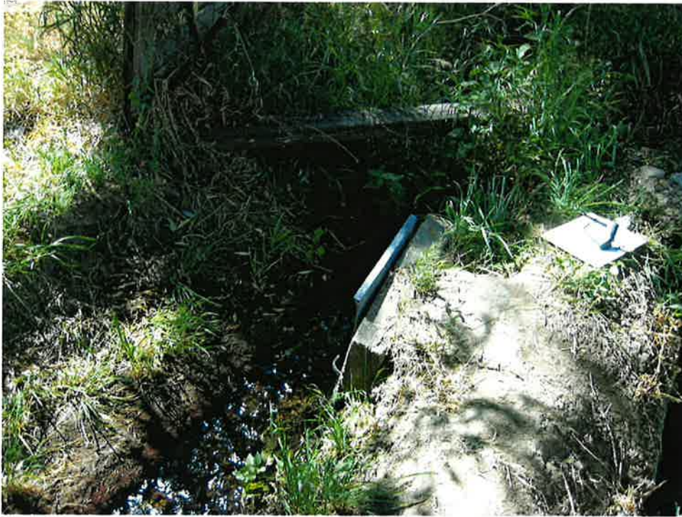
Looking at headgate where water diverts from the main ditch system to the claimed POU (csaxton).
