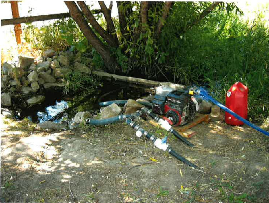
Pump that diverts water from the ditch system. Not an actual POD since it is diverting from a ditch (csaxton).
