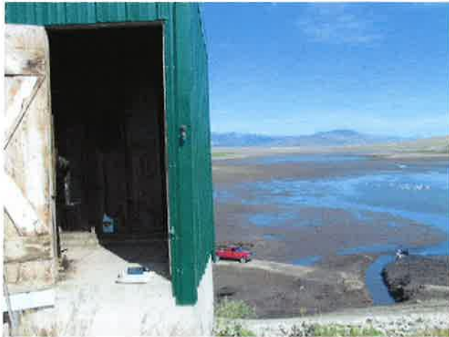
Photo 4. Release gate at Chesterfield Reservoir.
