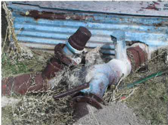
Photo 6. Looking north. Close-up of the pipes out of the 15 hp pump.
