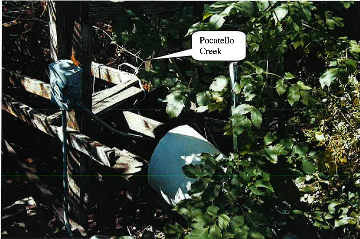
Small pump located under white metal half dome cover. Location of pump actually on the Hamlin property. Looking South (csaxton 9/26/01).
