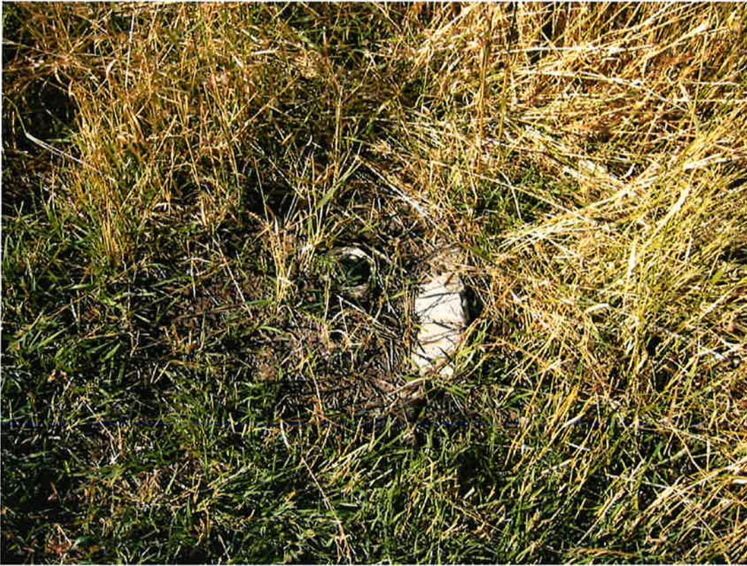
Looking at riser that can be opened to divert water to Jeffs Matkins place. (csaxton).
